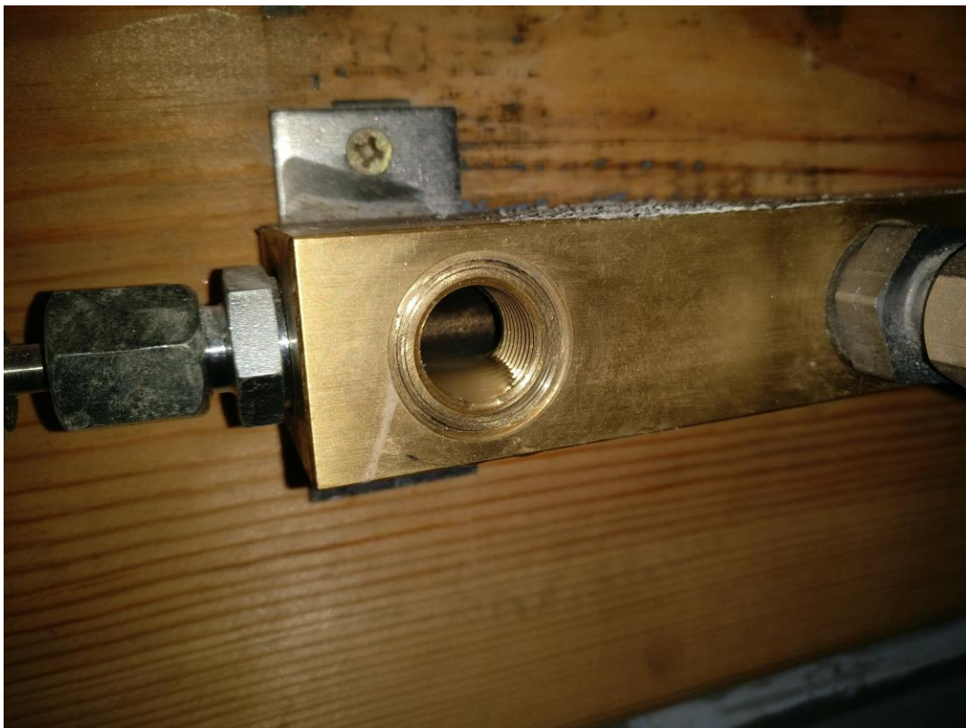
Figure 9 - Photo showing the water in the manifold blocks
