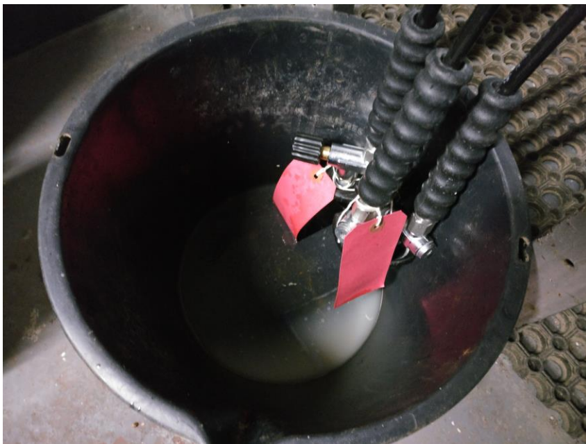
Figure 5 - A bucket catching the drips from the filling whips
