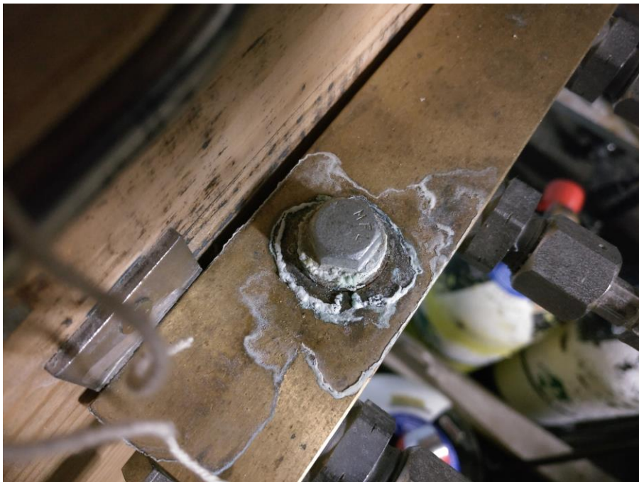
Figure 7 - Residue surrounding a leak on one of the manifolds
